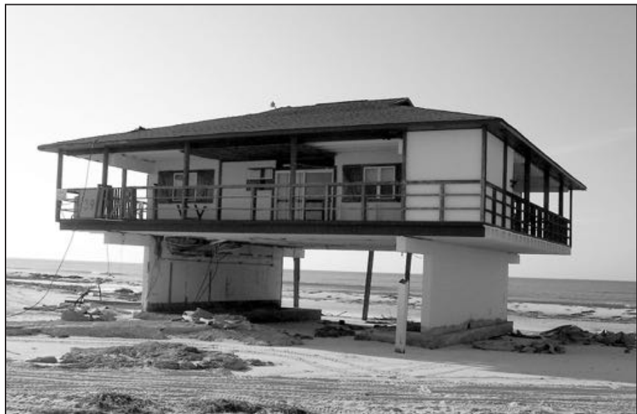
Figure 9. House elevated on shore-perpendicular shear walls. This design approach is risky for low-rise buildings since lateral out-of-plane loads (wind and flood acting on the faces of the shear walls) can be large and special design considerations and detailing are required.
