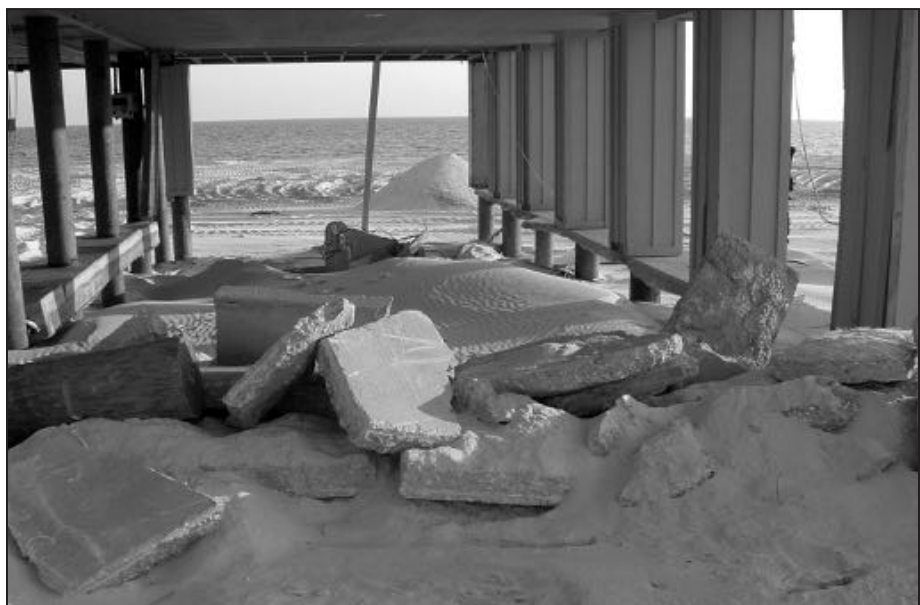
Figure 12. NFIP-compliant, unreinforced slab broke apart and performed well.
