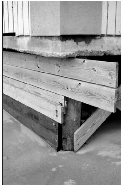
Figure 15. Shore-parallel timbers attached to a pile foundation were intended to act as a bulkhead, but constitute an obstruction and are prohibited.
