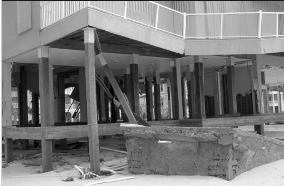
Figure 18. Movement of a spa likely caused failure of two piles supporting an elevated deck.
