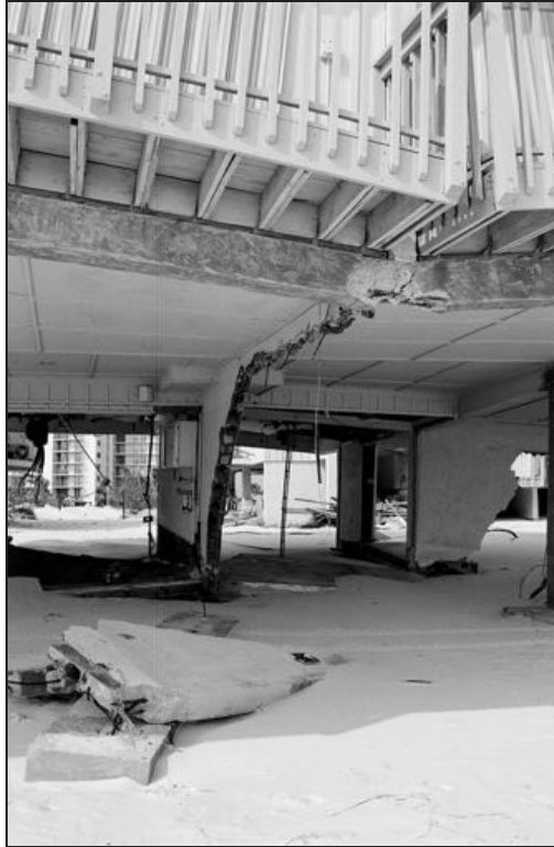
Figure 10. Failure of shore-perpendicular (and shore-parallel) solid foundation walls, and of beam and floor system supported by the shore-perpendicular wall (pre-FIRM structure)
