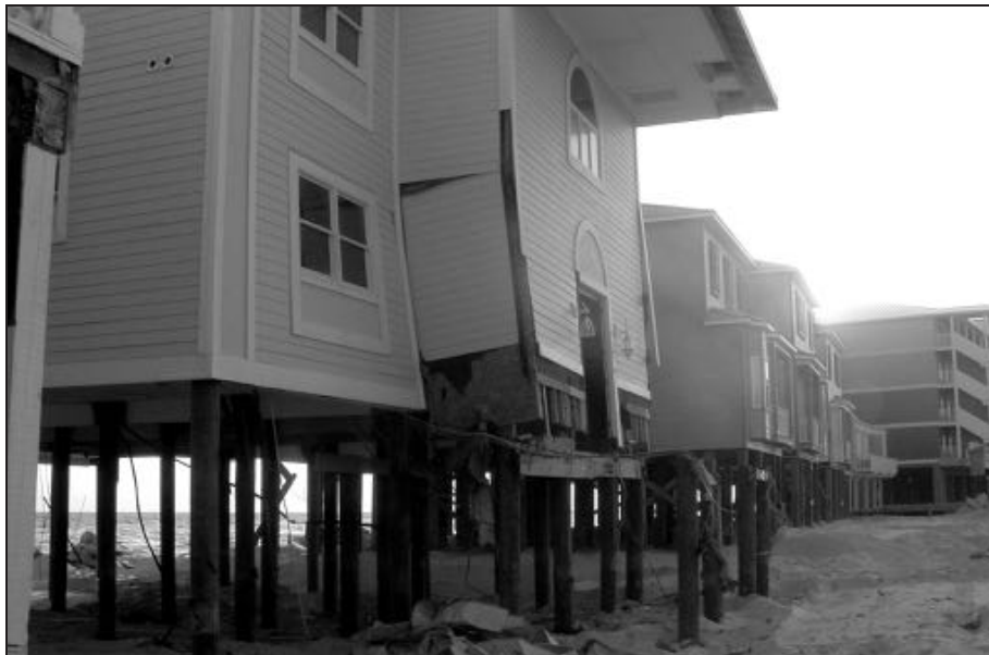
Figure 1. Stairs did not break away cleanly, resulting in damage to the elevated building.
