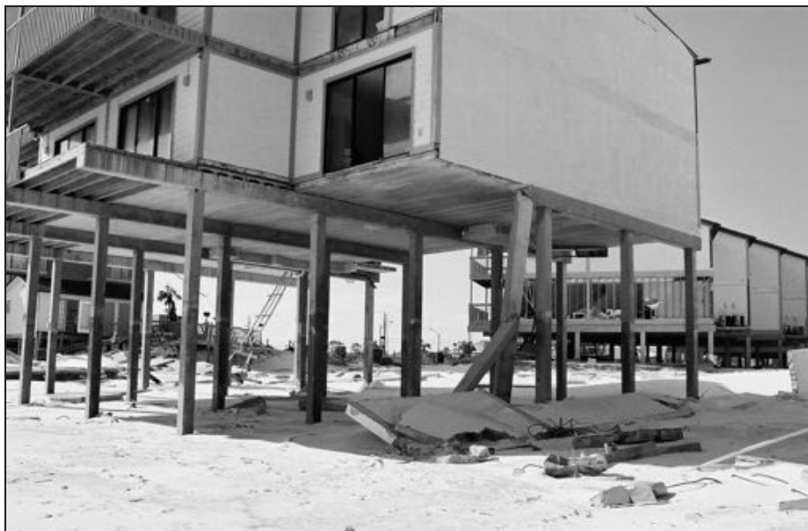
Figure 16. Shore-perpendicular reinforced masonry wall failed and collapsed into the foundation of an adjacent building, contributing to failure of the corner foundation piling and pile cap/beam.
